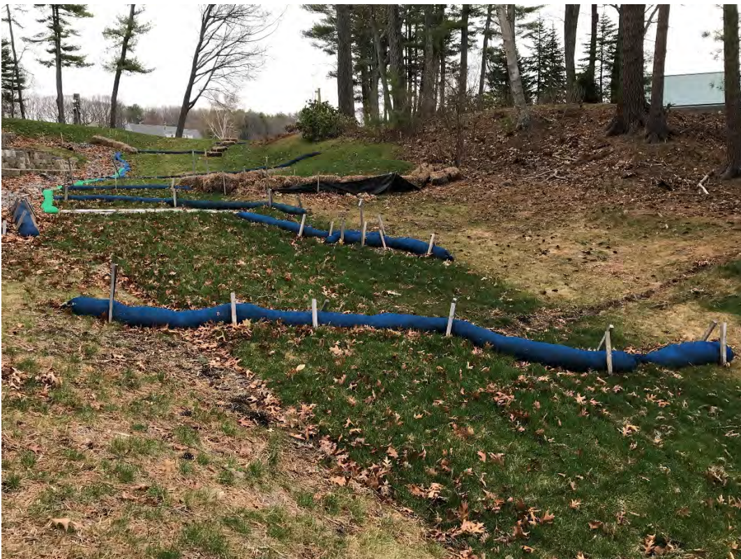
Fig 10: Slope below the manhole at Gundalow Landing/east side of the bay. Viewing east. (04-14-21)
