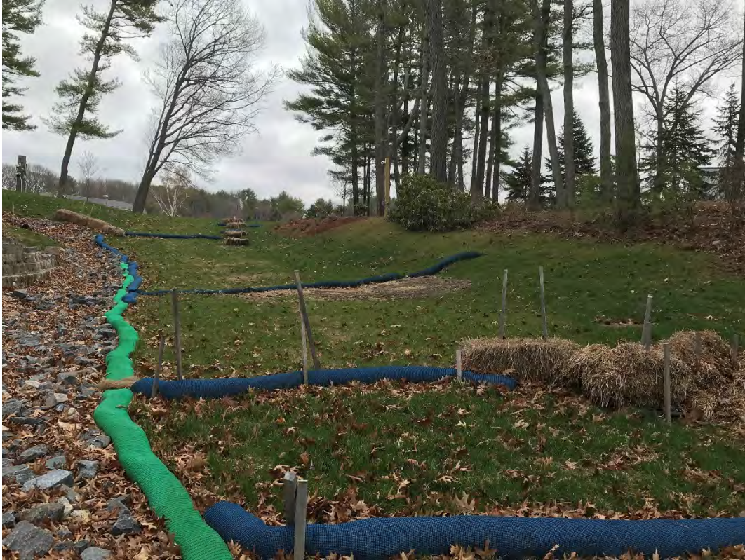
Fig 9: Slope above the manhole at Gundalow Landing/east side of the bay. Viewing east. (04-14-21)
