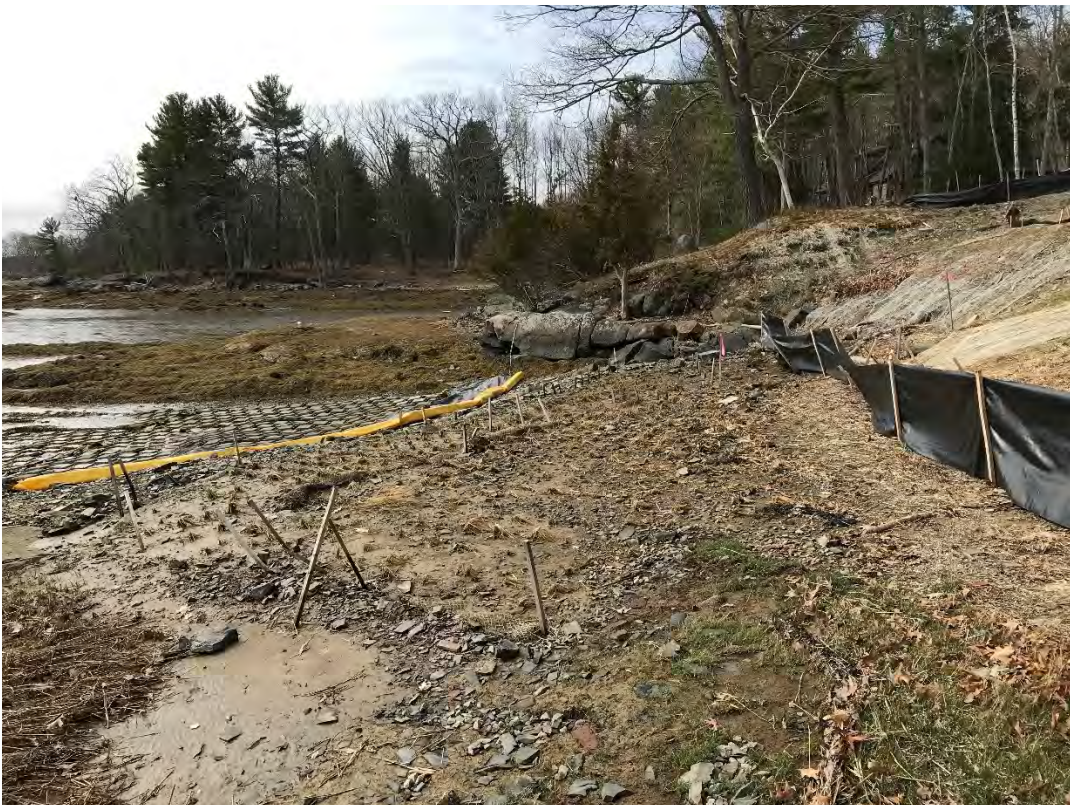
Fig 4: Toe of the slope and salt marsh restoration at the west side of the bay. Viewing south. (04-14-21)
