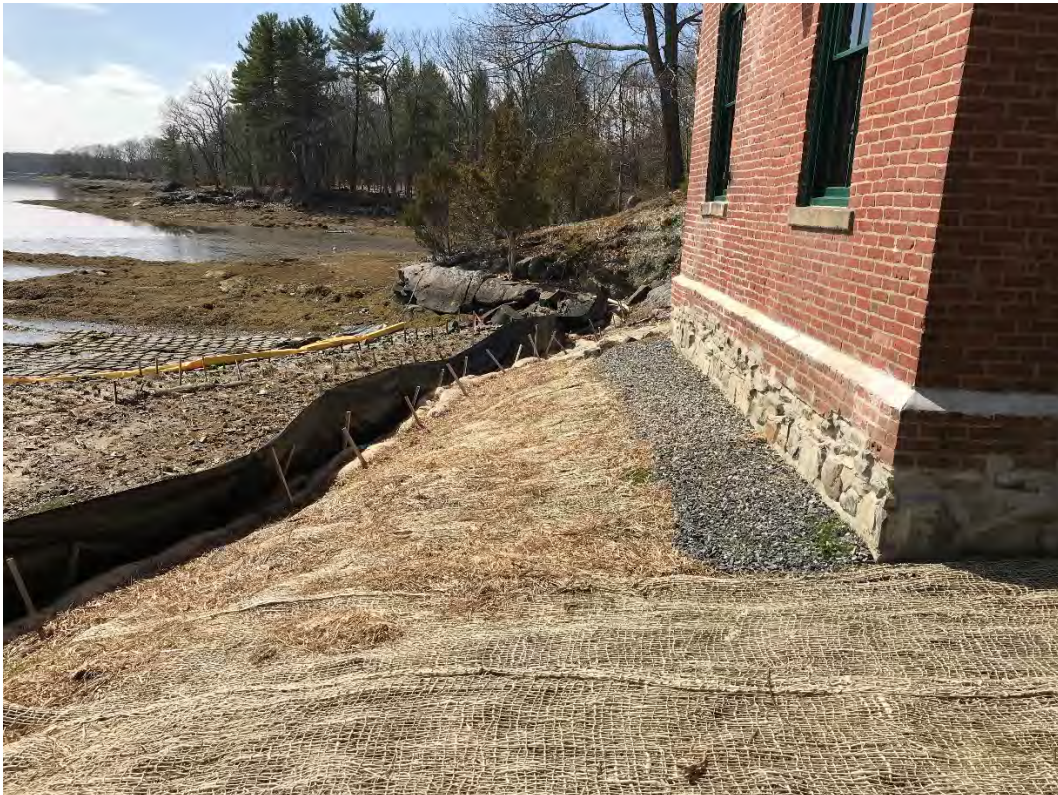
Fig 2: Slope between the cable house and salt marsh restoration at the west side of the bay. Viewing south. (04-14-21)
